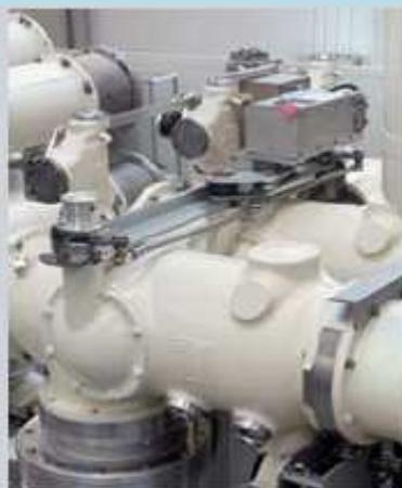
High voltage GIS
